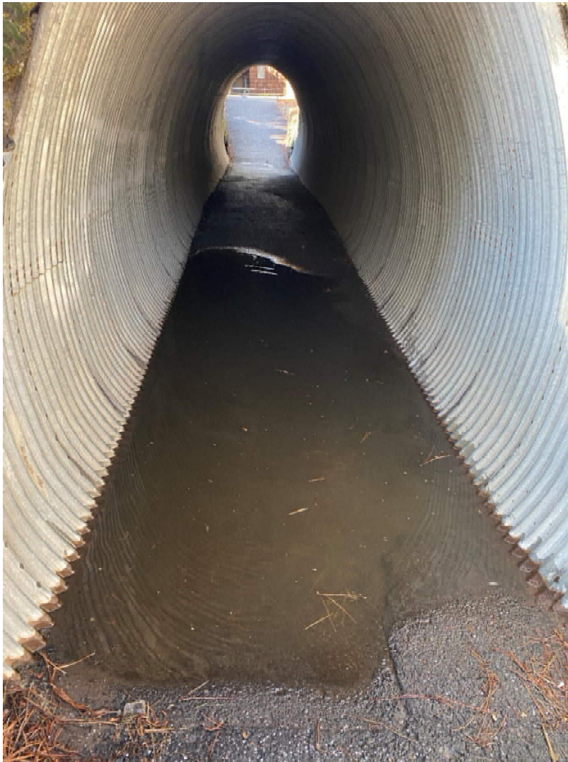
Flooding Inside Tunnel
