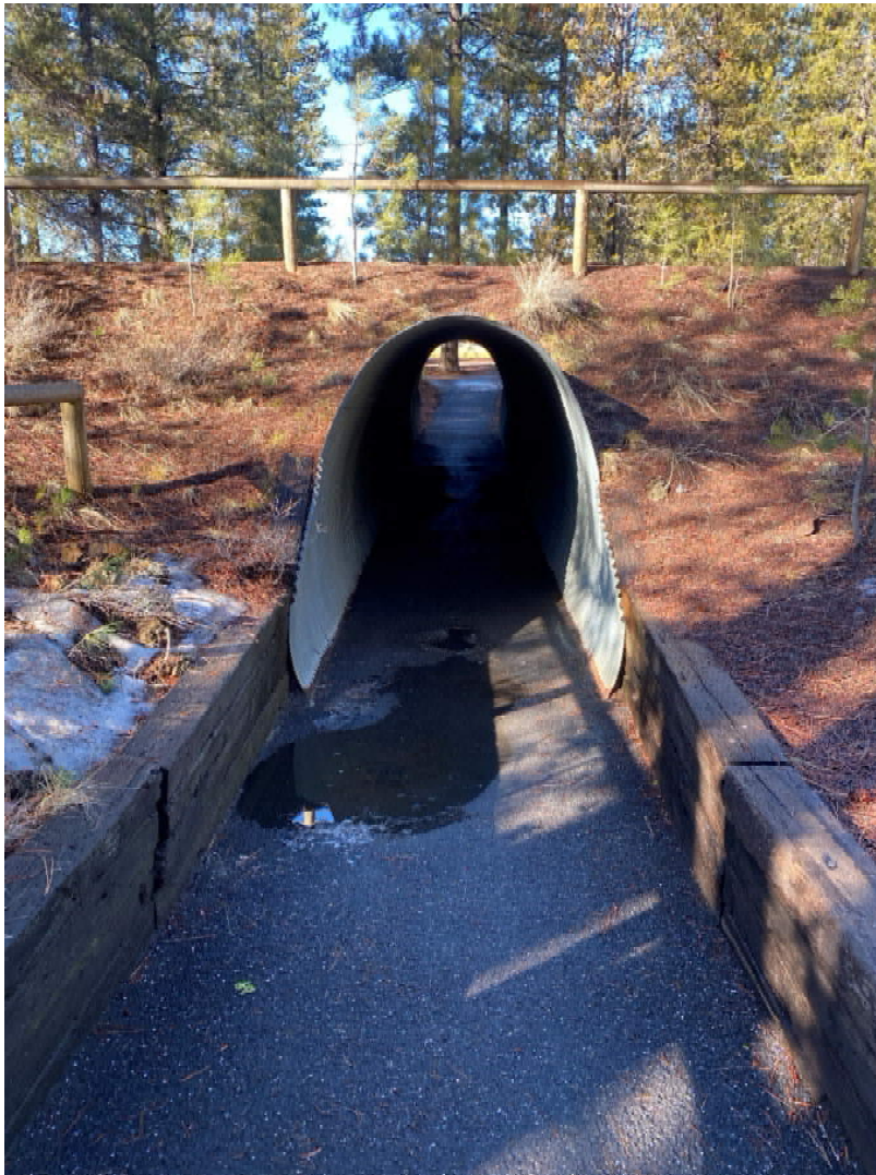
Flooding Outside Tunnel Entrance
